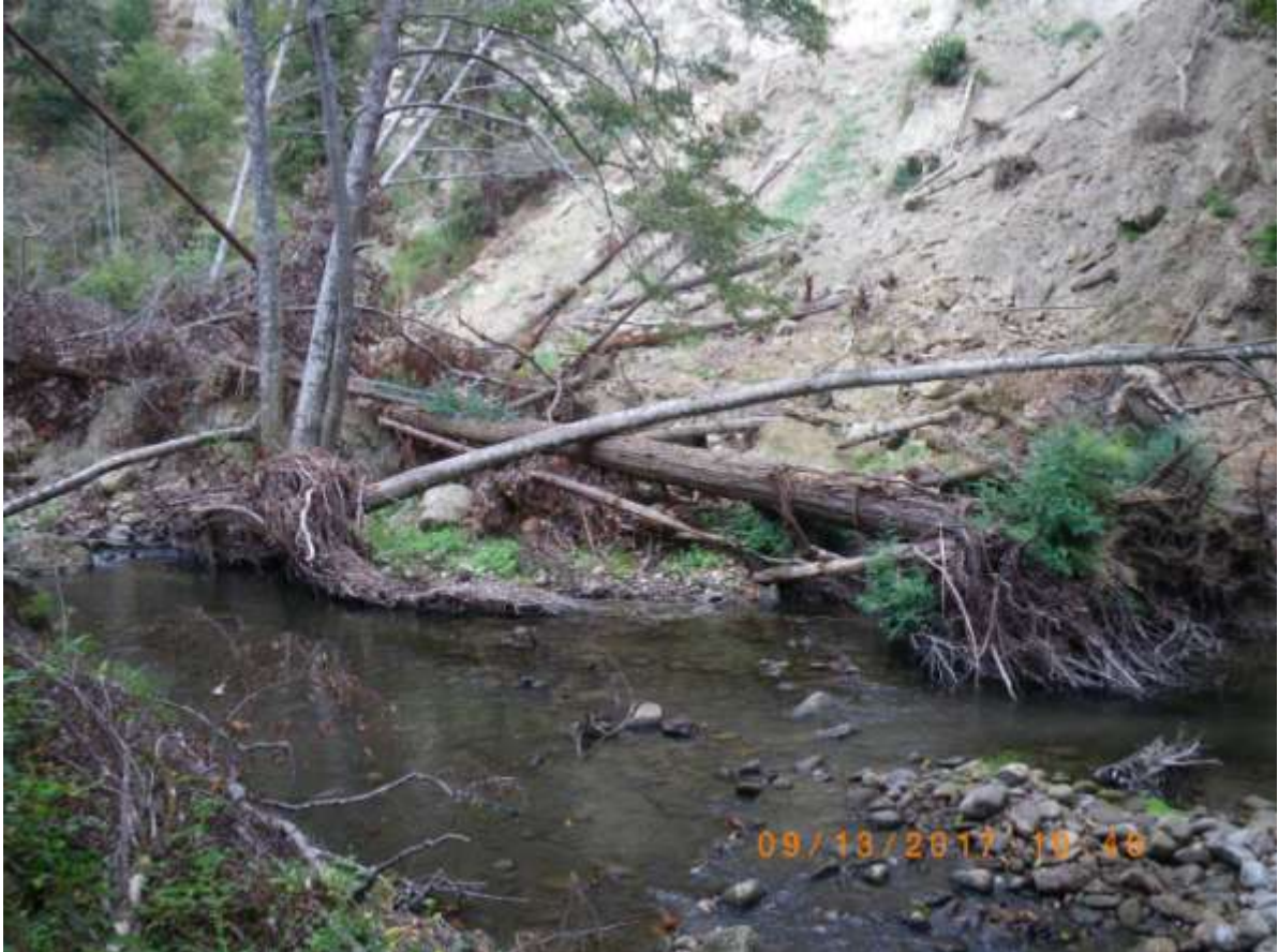
Sampled Pool in Mainstem Soquel Creek Site #10, Adjacent Large Landslide Activated by Heavy Rainfall
