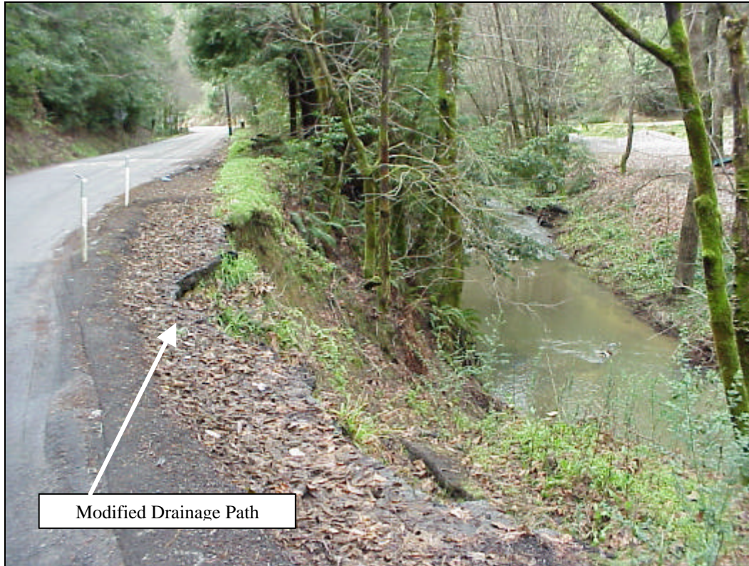
Figure 2.1. Road Shoulder and Streambank Failure in Road-confined Inner Gorge Area of Zayante Creek. (Failure is likely due to sheet flow erosion and saturation of streambank material resulting from a plugged culvert.)
