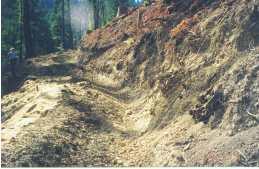
Figure 4.1: Recently Built Timber Harvest Road in the Fritch Creek Drainage that was cited for a grading violation by Santa Cruz County.
