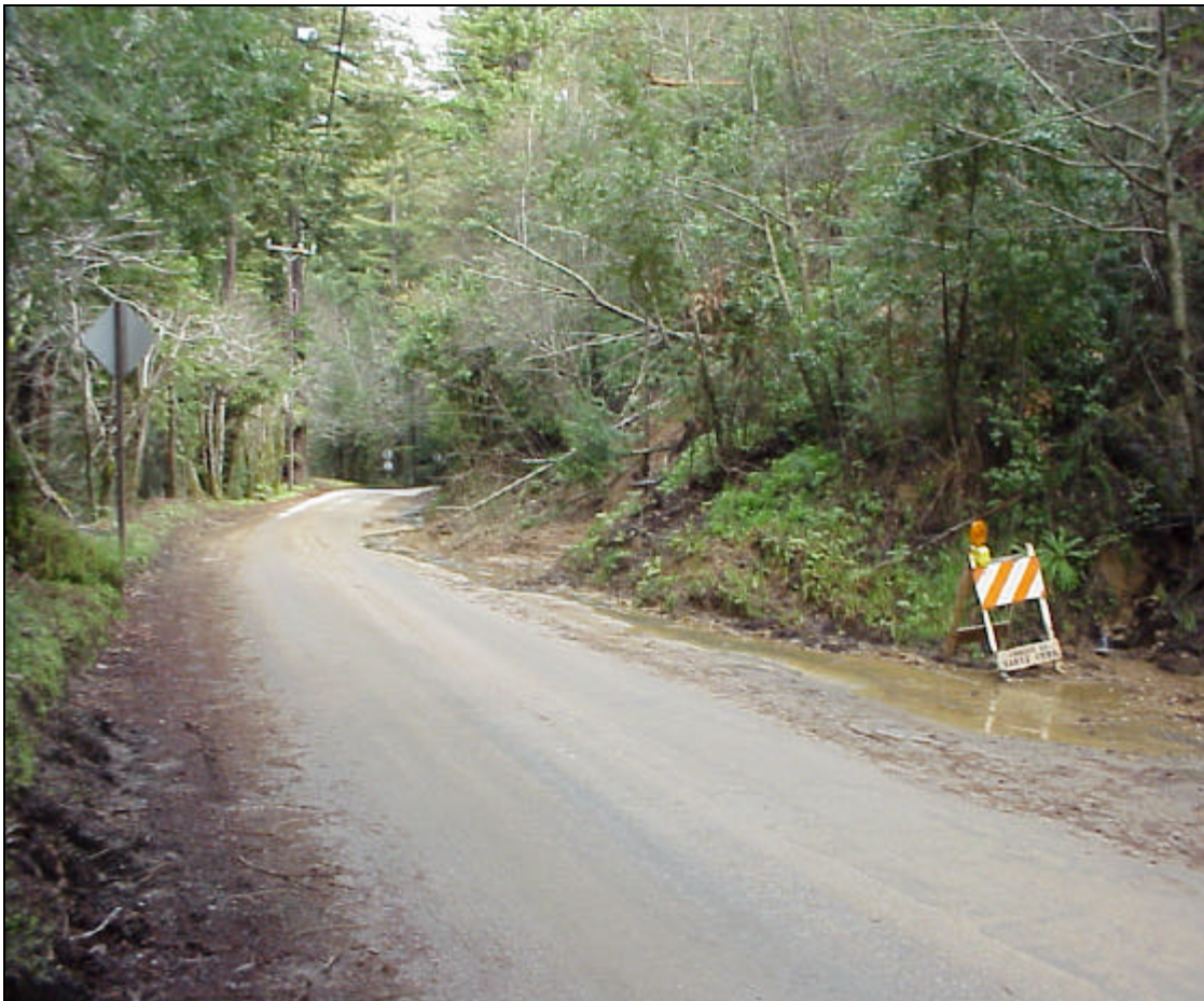
Figure 2.2. Roadcut Failure and Landslide Over East Zayante Road. Inside ditch and cross culvert are overwhelmed by the sediment load, which forces sheet flow over the road surface.
