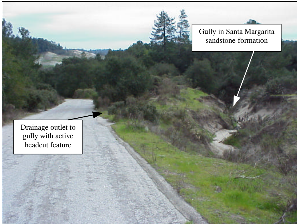
Figure 3.5: Gully Development Adjacent to McEnery Road
